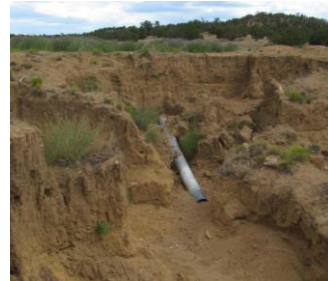
Erosion on Coyote Creek bank
