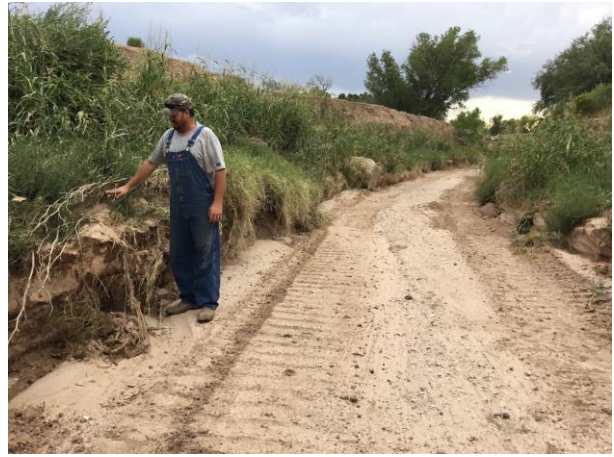
An example of a 4-foot cut caused by and extreme rain event
